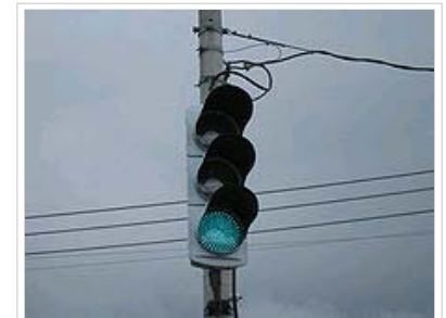
Traffic light using LED
